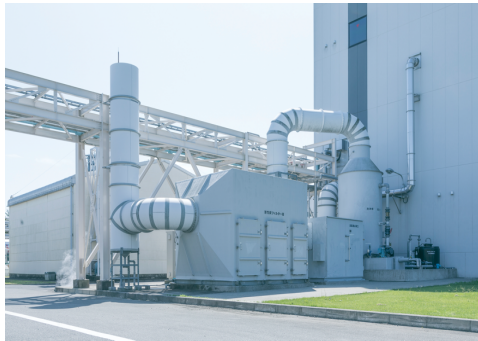
Deodorizing System (Itakura Factory)
