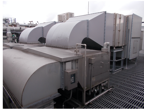
Deodorizing System (R & D Center)
